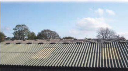
Figure 1: The ridge in the foreground has the maximum possible number of ridge vents - but provides much less than the required outlet.
